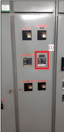
1) HVAC General Circuit Break
